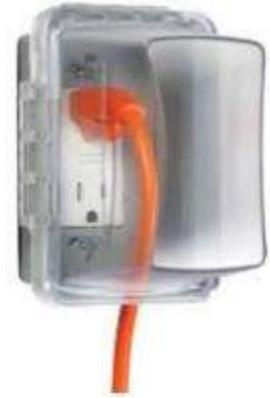
Outdoor outlets require covers approved for wet locations and must be marked extra duty .
